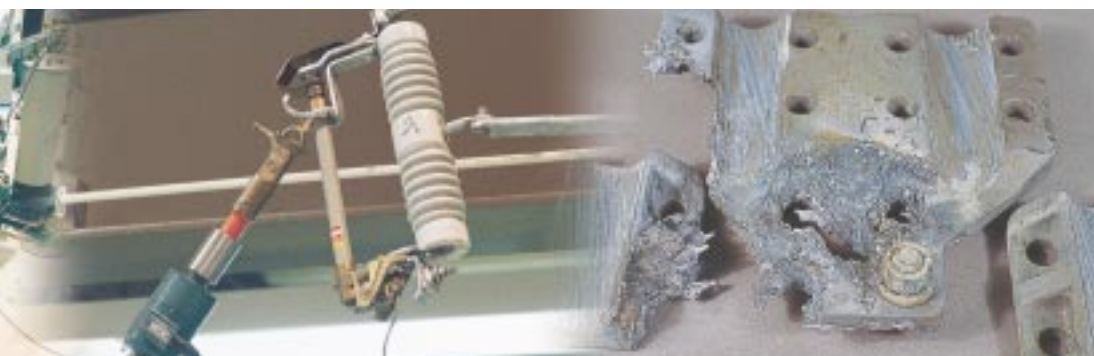
Measuring the physical force used by linemen to close a fuse (pressure on the porcelain can cause it to break).
